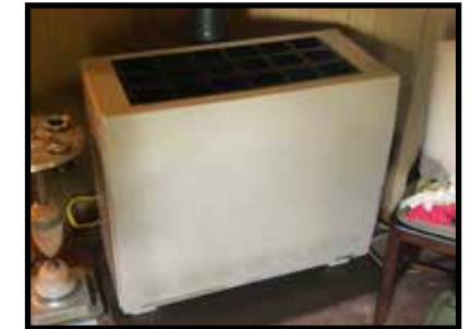
2012 Empire LP heating stove, bought new from Hechler Hearth
