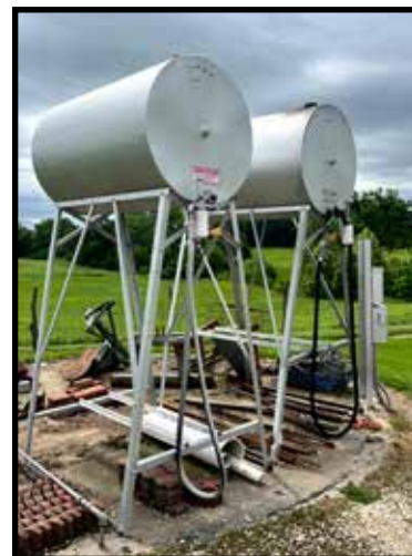
2, 500 gallon fuel tanks & stands; 1 gas & 1 diesel
